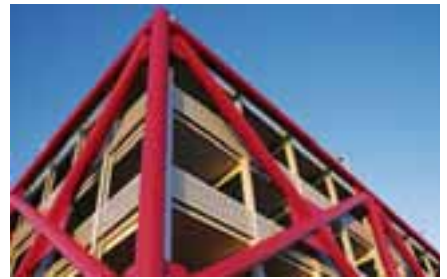
... Corrosion protection coatings
